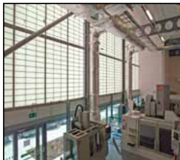
KALWALL PROVIDES THE ADVANCED MANUFACTURING RESEARCH CENTRE AT ROTHERHAM WITH GREAT AMBIENCE
